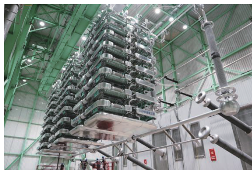
图3 CLCC阀塔 Fig. 3 Valve tower of CLCC
